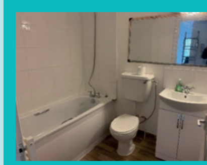
New Bathroom at Downs Rd. This is one of 2 new bathrooms we installed in 2022/23
